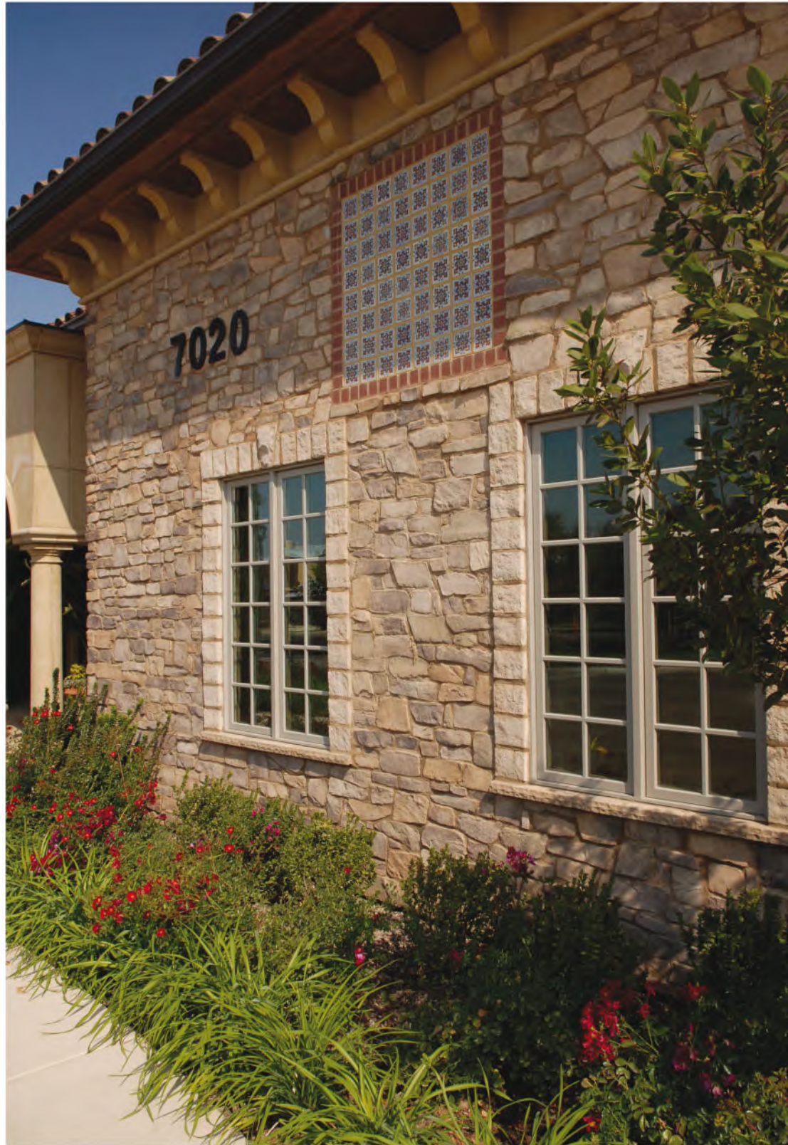
Foundation treatments that obscure the required termination of manufactured stone above grade can include a bed of stones placed adjacent to the wall along with a landscape area beyond that can screen the transition.
