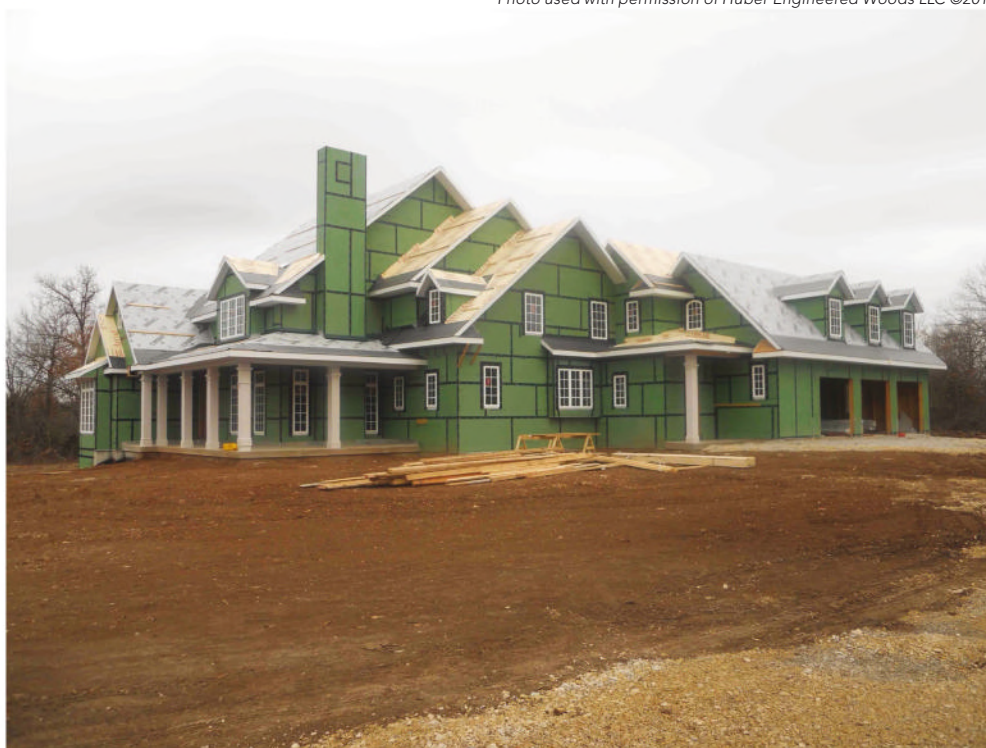
Inadequate strength may not lead to dramatic failure, but it could lead to a compromised structure. There is more to structural requirements than framing.
